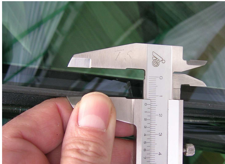
White Lines at the Edge Bond of a Solar Protection Glass Pane
